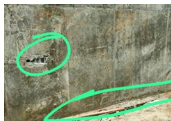
Gambar 1 Contoh defect di lapangan ( Major Honeycomb pada dinding lantai basement)
